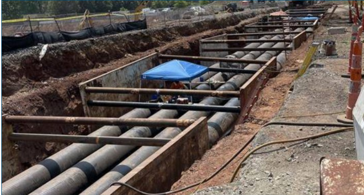
Princeton University Steam to Hot Water Conversion
